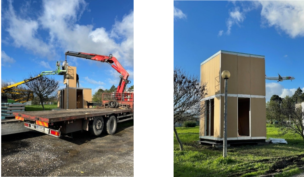
Figure 19. Pilot Construction – LNEC Campus – Reassembly of the Prototype taken to test on the seismic table.
